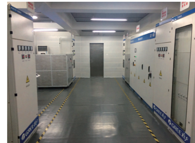
PV Power Room
